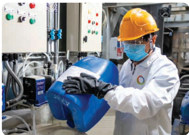
FSE Environment's HVAC water treatment service is well-known for the professionalism in the industry with over 40 years of history.
